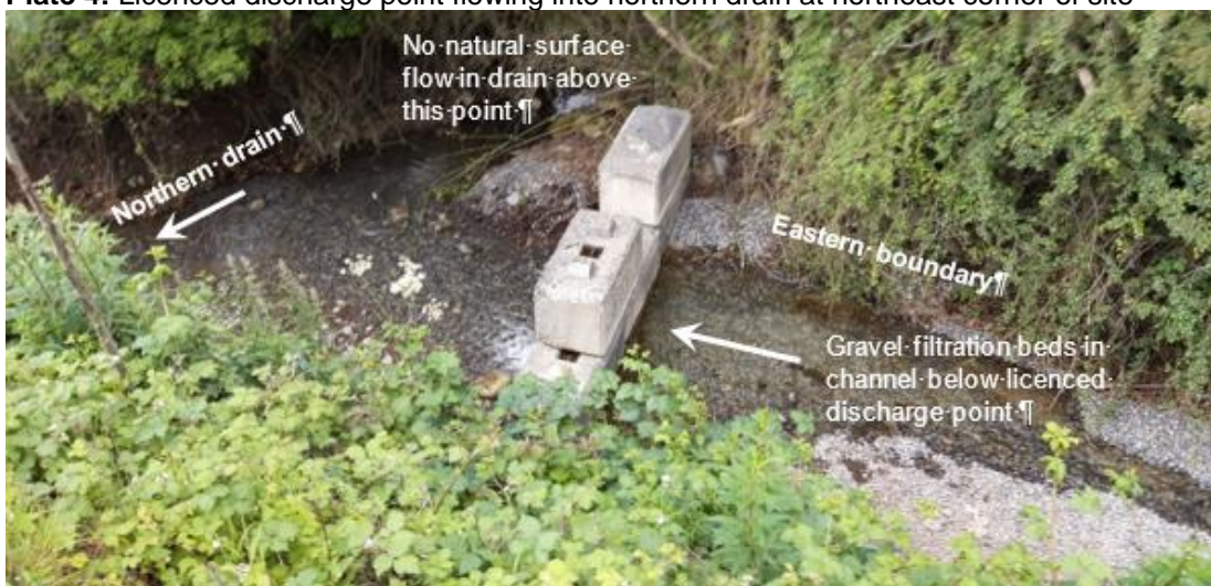
Plate 4: Licenced discharge point flowing into northern drain at northeast corner of site
